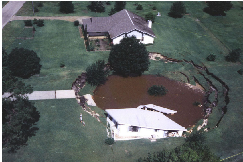
A home falls into a large sinkhole in Florida. CREDIT: SOUTHWEST FLORIDA WATER MANAGEMENT DISTRICT
